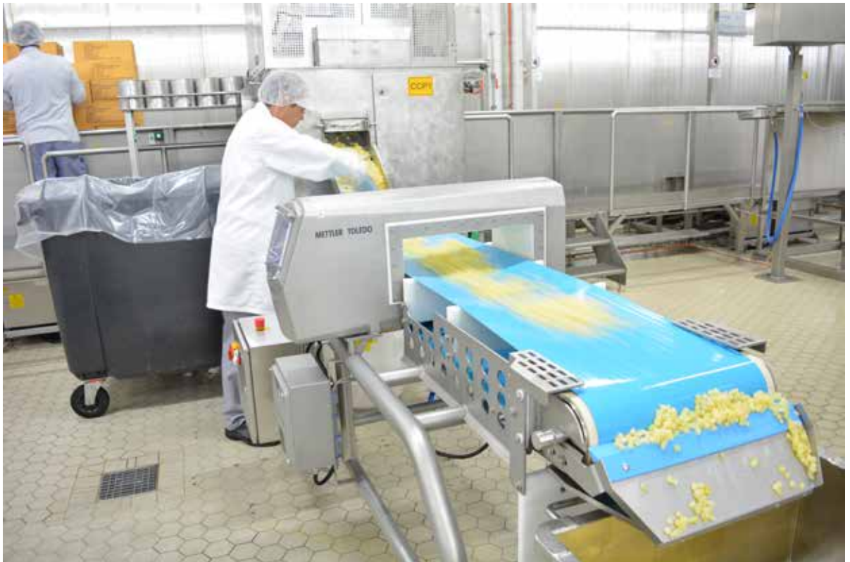
When metal is detected, the product is ejected from the process by reversing the conveyor belt. This approach improves process reliability at Zentis, and ensures only raw goods that are completely free of metal are processed further, protecting its products and brand.
